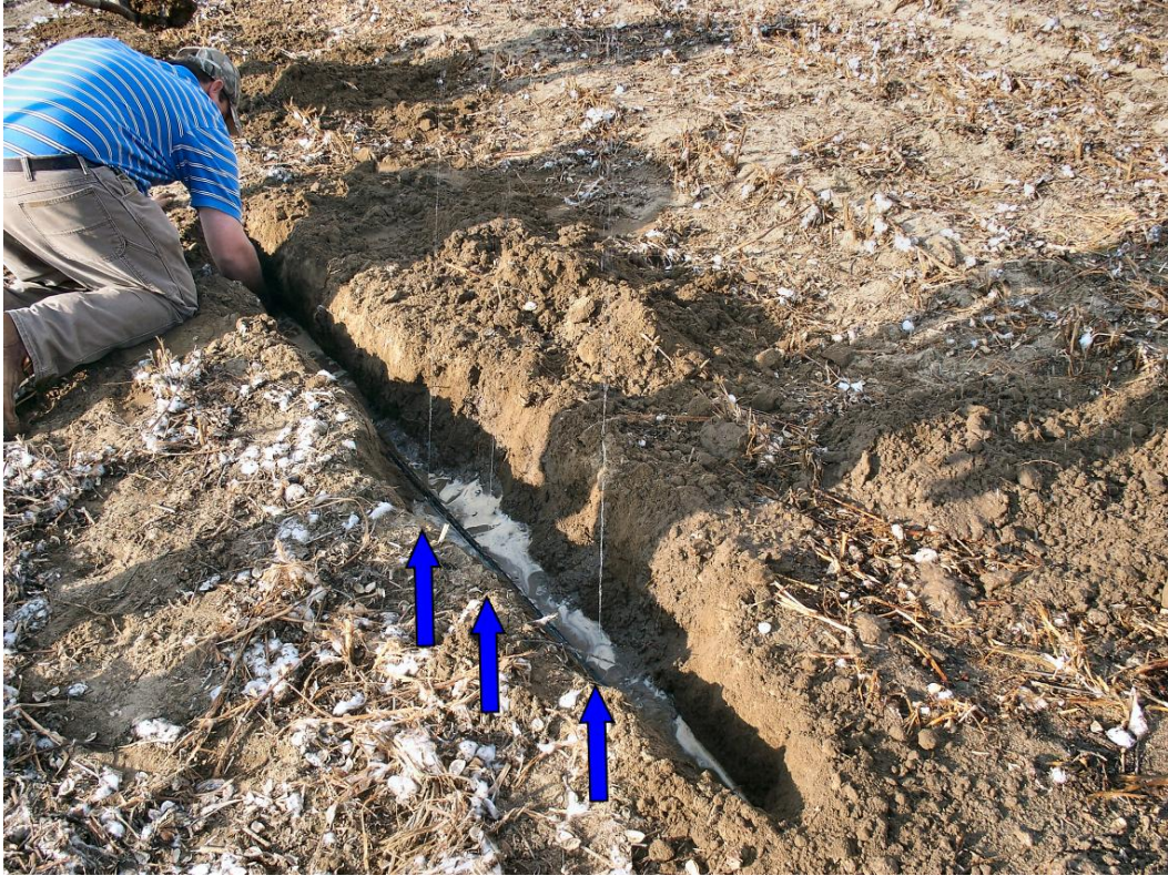
Jay discovered leaks in one section of the deep tape (10"-12") in the SSDI project area near the front of the Park (see blue arrows). Mice are to blame (we think).
