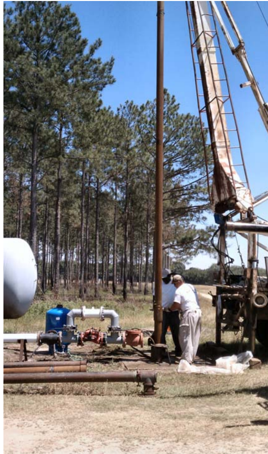
Pulling the pump from one of SIRP's wells to repair the wiring.
