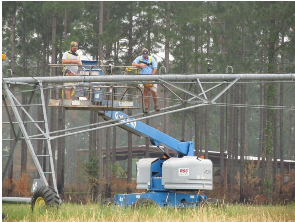
Jay and Matt installing new regulators and sprinklers on center pivot system.
